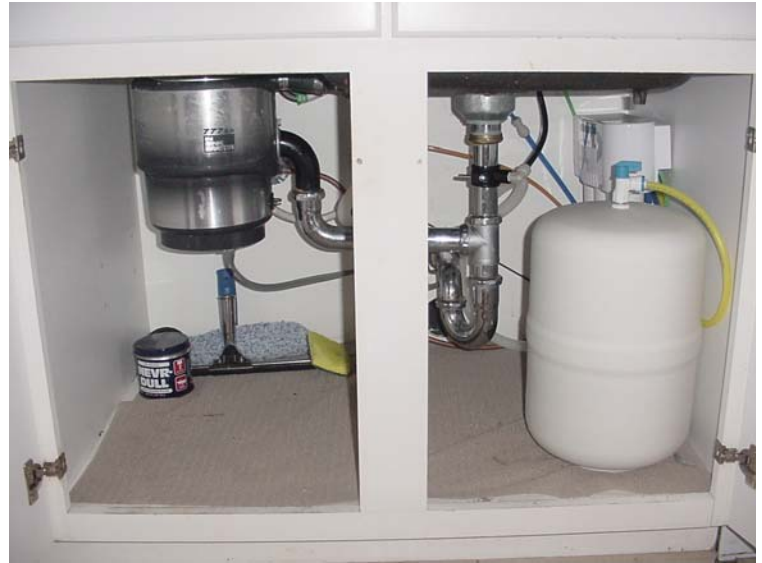
Haleiwa (Sunset Beach) Installed 6/7/07
