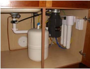
Ewa Beach (Haleakea) Installed 8/28/08
