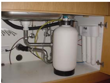
Honolulu 96821 (Aina Haina) Installed 10/24/03
