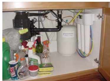
Honolulu 96825 (Hawaii Kai-Peninsula Villas) Installed 2/9/09
