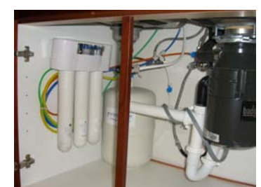
EWA BEACH (Latitudes) Installed 8/15/08
