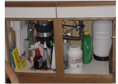
Honolulu 96826 (Mc Cully Area) Installed 5/20/03
