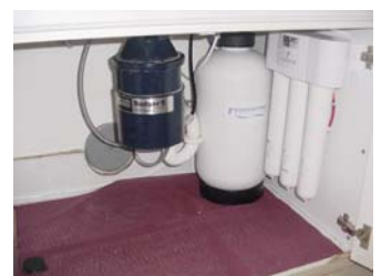
EWA BEACH (Ali'i Cove) Installed 12/1/05
