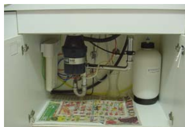
WAIPAHU (Sea View) Installed 4/5/04
