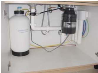
EWA BEACH (Prescott II) Installed 10/5/05
