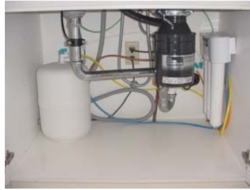
AIEA (Aiea Park Place) Installed 12/6/07
