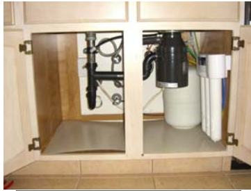
Kapolei (Makakilo-West Park) Installed 12/18/08
