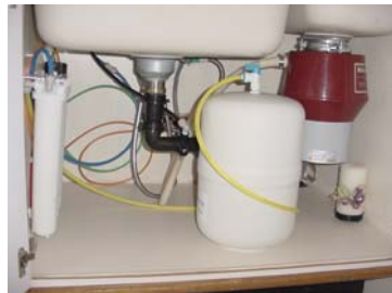
Honolulu 96817 (Honolulu Tower) Installed 11/5/07
