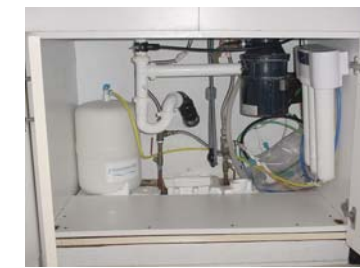
KAILUA (Keolu Hills) Installed 5/31/08
