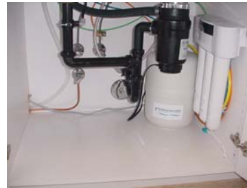
Ewa Beach (Ocean Point —Town Homes At Fairways Edge) Installed 12/28/07
