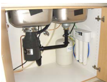
Kapolei (Makakilo-Waikoloi) Installed 4/11/09
