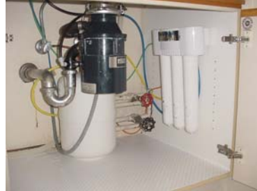
Honolulu 96826 (McCully-Crystal Park Apts.) Installed 1/26/09
