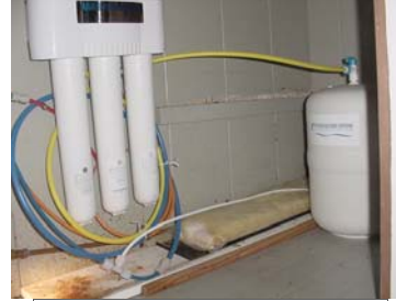
Honolulu 96821 (Aina Haina) Installed 2/4/09
