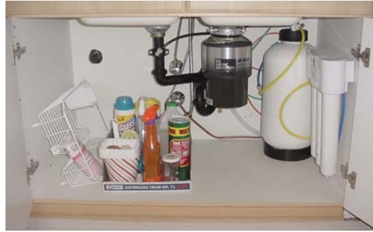
SQC3 Reverse Osmosis System
