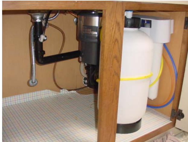
SQC3 Reverse Osmosis System
