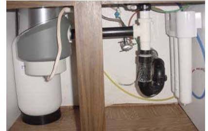
SQC3 Reverse Osmosis System
